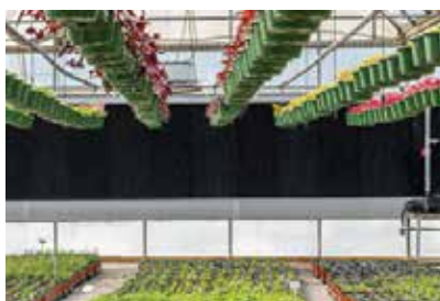
EVAPORATIVE PAD COOLING SYSTEMS
