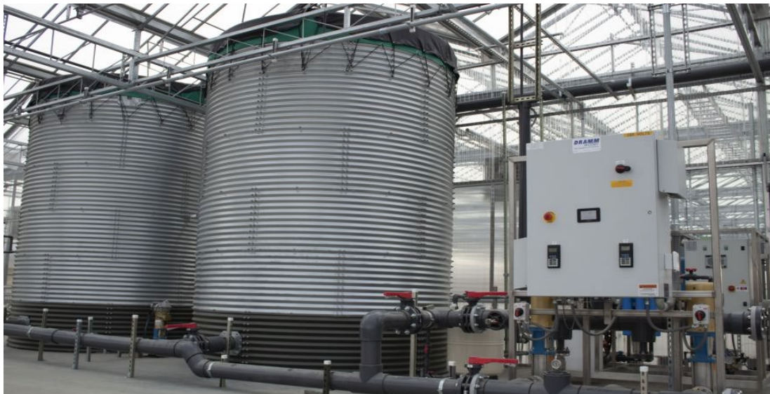
Prides Corner Farms is updating its water circulation process to allow treated water to be held in ready-to-go silos.
